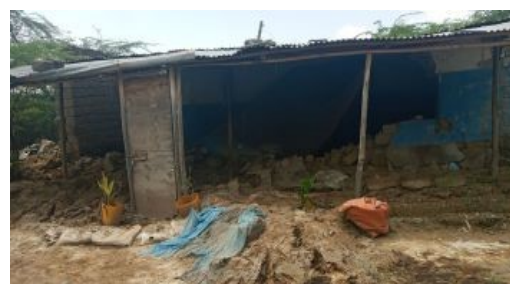
Figure 5 House demolished by flooding. Photo credit: OCHA
