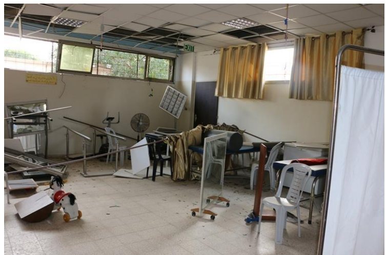
Palestine Avenir for Childhood Foundation (PACF) – Cerebral Palsy Center exposed to severe damages due to an Israeli airstrike nearby the building. Photo credit: PACF
