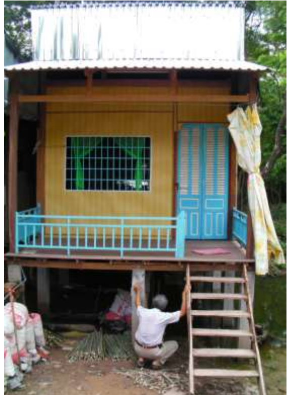
A regular visit paid by VNRC staff to construction site to ensure quality and progress of the work within project timeframe. Photo: Ben Mountfield
