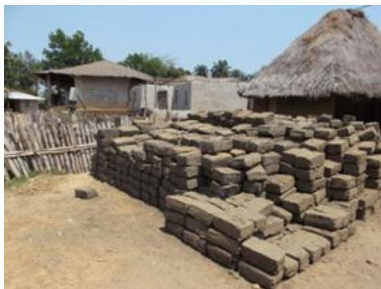
In April 2013, RDRT Shelter (SLRCS) supported reconstruction of burnt houses in Blama Gbannie, Bo District. Photo: SLRCS
