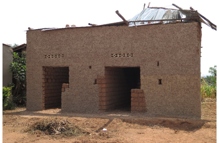
House with roof destroyed in Gatsibo district ©IFRC
