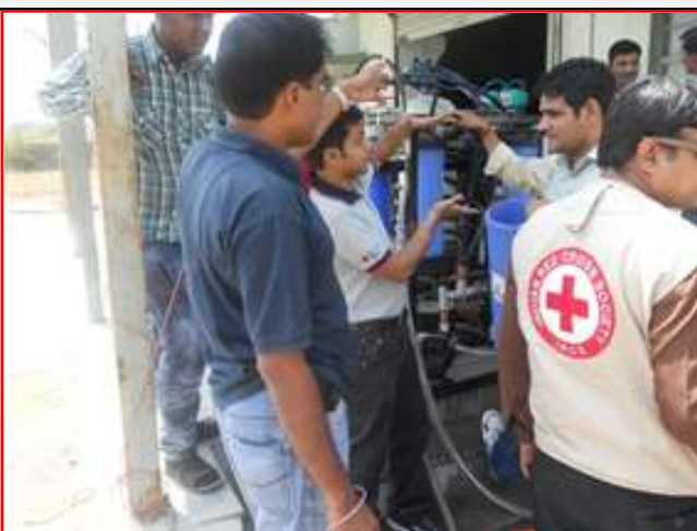
Installation of a water purification unit in Suigam village by the Gujarat branch of IRCS.
