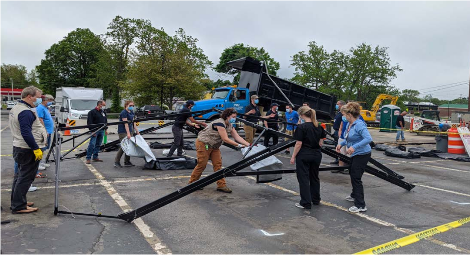
International Medical Corps logistics experts deploy emergency field units at Brockton Hospital in Brockton, MA.
