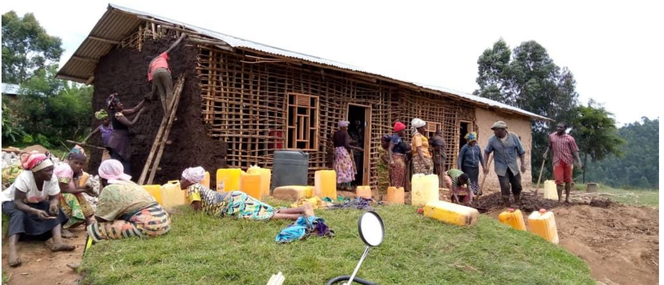
International Medical Corps' protection program mobilized in Masereka to rehabilitate a building that will serve as a women and girls' safe space.
