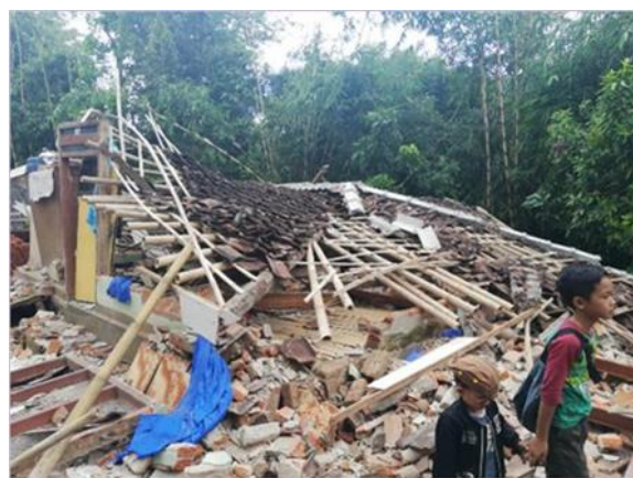
A completely damaged house in North Lombok. (Photo: PMI)
