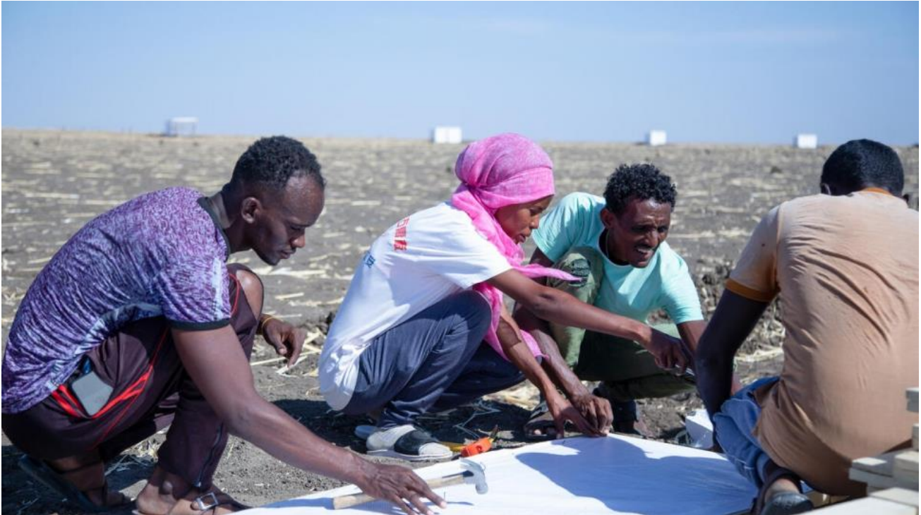
Mihret, 25, an Ethiopian refugee and engineer, oversees construction at a site in Tunaydbah settlement, Sudan. © UNHCR/Ahmed Kwarte
