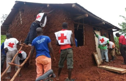
Rwanda Red Cross volunteers constructing house and toilet for the most vulnerable family photo/RRCS
