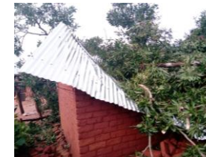
Damage to housing in Yamodo centre ©OIM Chad 2021/ Abdoulaye Samson
