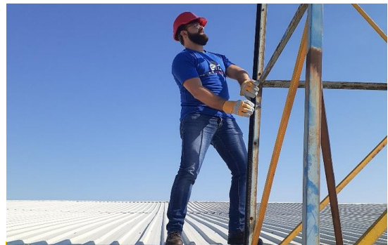
ETC Senior IT Associate Omar Mardini makes upgrades to communications infrastructure at a WFP warehouse evacuation site in Qamishli.
