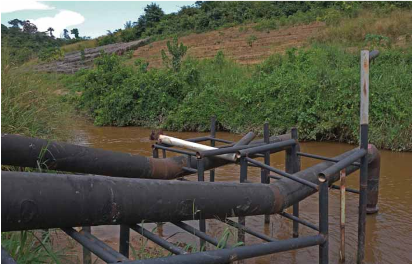
The intake of the REGIDESO's water treatment plant on the Lukaya River, where UNEP plans to pioneer the DR Congo's first integrated water management initiative
