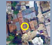
GRADE 4: VERY HEAVY DAMAGE ; Part of building structure collapsed, such as part of roof or one or more fallen walls
