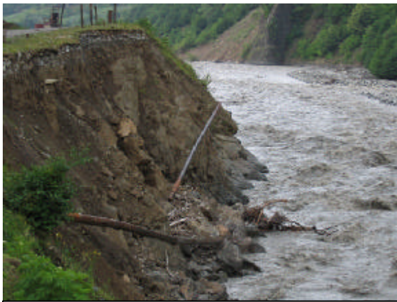
Destroyed water supply system in Oni region
