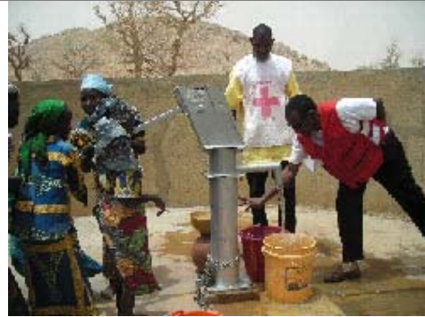
A water pump is restored in Zinder, Niger, as part of the Red Cross/Red Crescent WatSan project. Kinvi/International Federation
