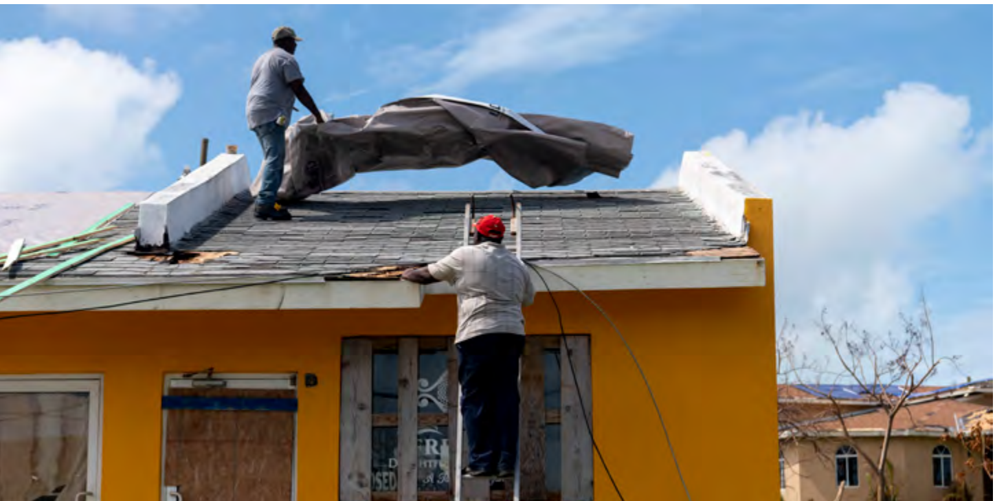
Local residents of Marsh Harbor on Abaco Island cover a roof affected by the hurricane with tarp. Photo: UN/OCHA/Mark Garten, September 2019
