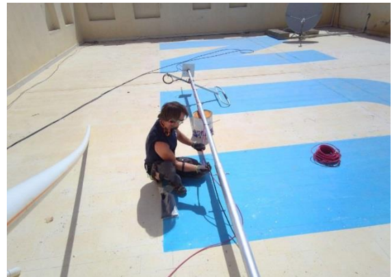
ETC telecommunications specialist relocating the COMCEN in the UNICEF building in Sa'ada.
